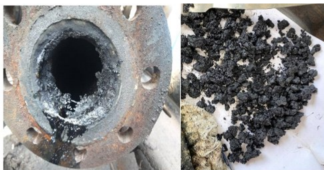
Fig. 1: Tar deposition in heat exchangers tubes.
