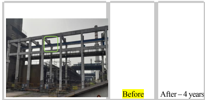
Fig. 1: Grab bucket monorail beam life Comparison : Corrosion, Quenching Steam
