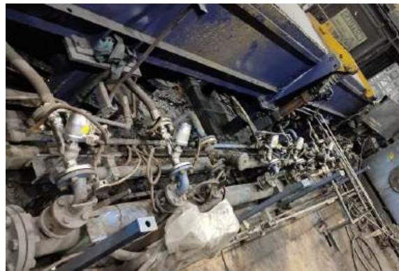
Fig. 1: Fast response valve at water box
