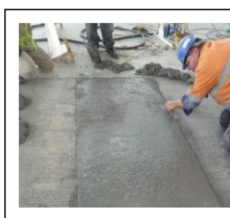
Fig.2 No cold Joints
