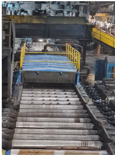
Fig. 1: Primary descaler hood
