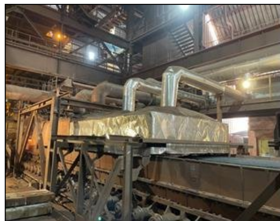
Fig 2. Hot air for new hood drawn from tapping in main hot air line
