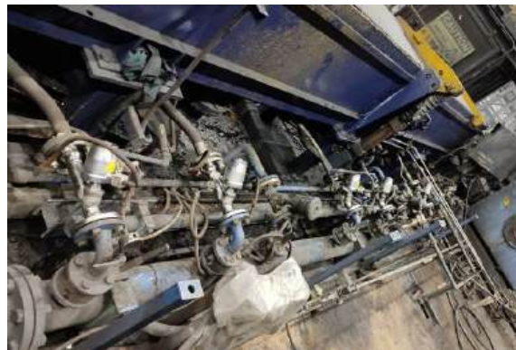
Fig. 1: Fast response valve at water box
